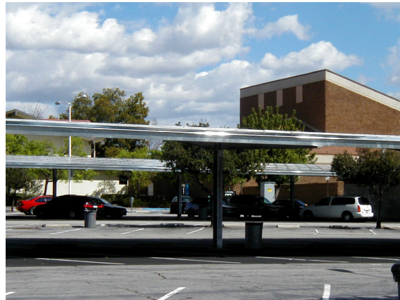
Photovoltaic cells in the parking lot of Pierce College transform solar energy into power for the energy-efficient campus.
