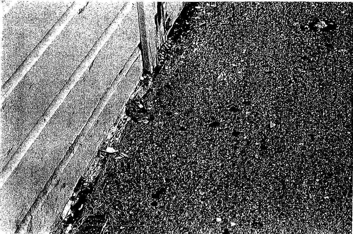
Paint Chips on Ground
