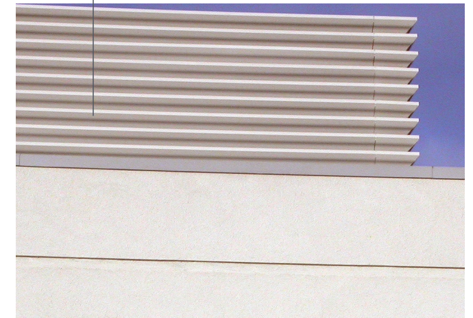
Lightweight enclosures define mechanical equipment
