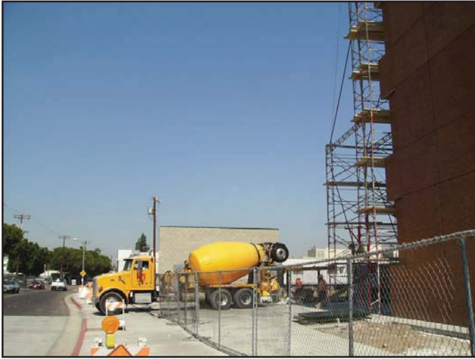
View 15: View from the intersection of W. 23rd Street and Grand Avenue looking northwest at LATTC's existing campus.
