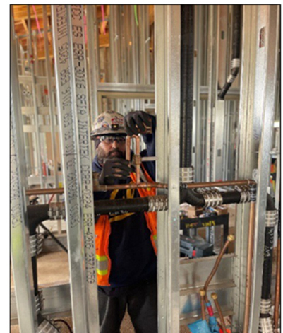
Bill Pena Apprenticeship: LA Trade Tech CMU Program Local: Plumbers Local 78 Contractor: Pan Pacific Project: Pierce College – Agricultural Educational Bldg.
